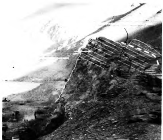
Fig. 8: Photograph showing the disposition of slip plane along the cut slope.
